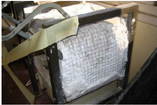
Photograph 01: Kiln with exposed lagging
