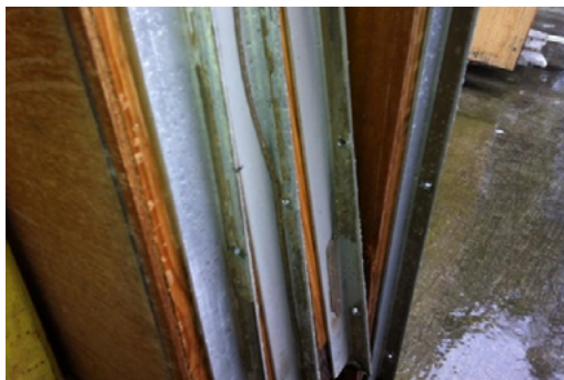
Photograph 03: Typical panels removed from demountable – red arrows show the location of the asbestos containing mastic on the aluminium frame of the panel
