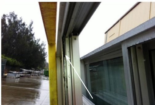
Photograph 07: Asbestos containing mastic in the groove of the window where the glass pane is inserted
