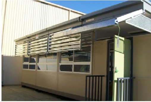
Photograph 01: Old system demountable showing typical wall panels and windows – view from front
